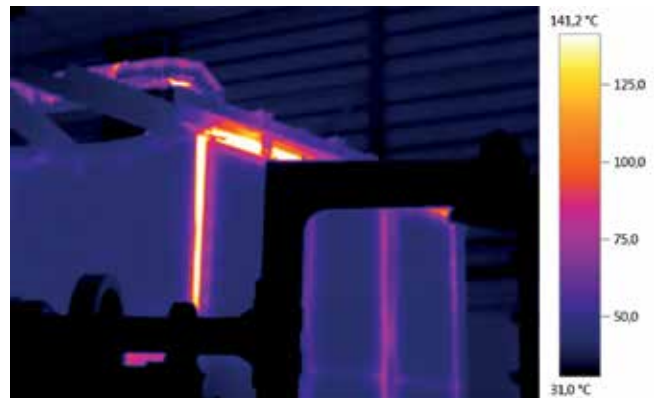
Industrial kiln with faulty insulation.
